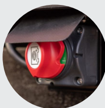
2. Battery shut-off switch
