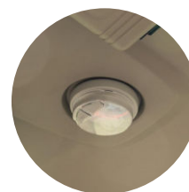
4. LED interior lighting
