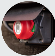
2. Battery shut-off switch
